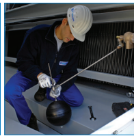
on site services
