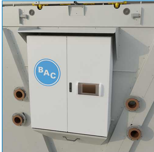
Panel de control
